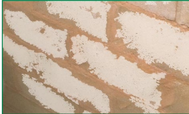
Figure 6.5 Remnants of asbestos on breeze blocks
